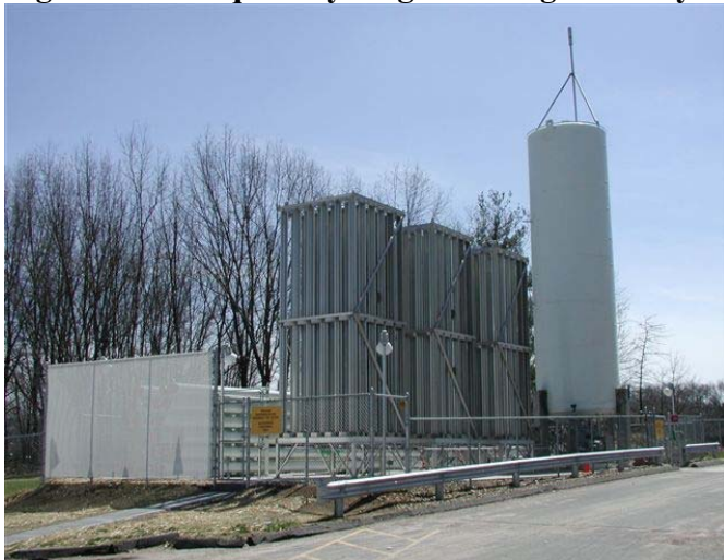
Figure VII– Liquid Hydrogen Storage Facility – UTC Power, South Windsor, CT
