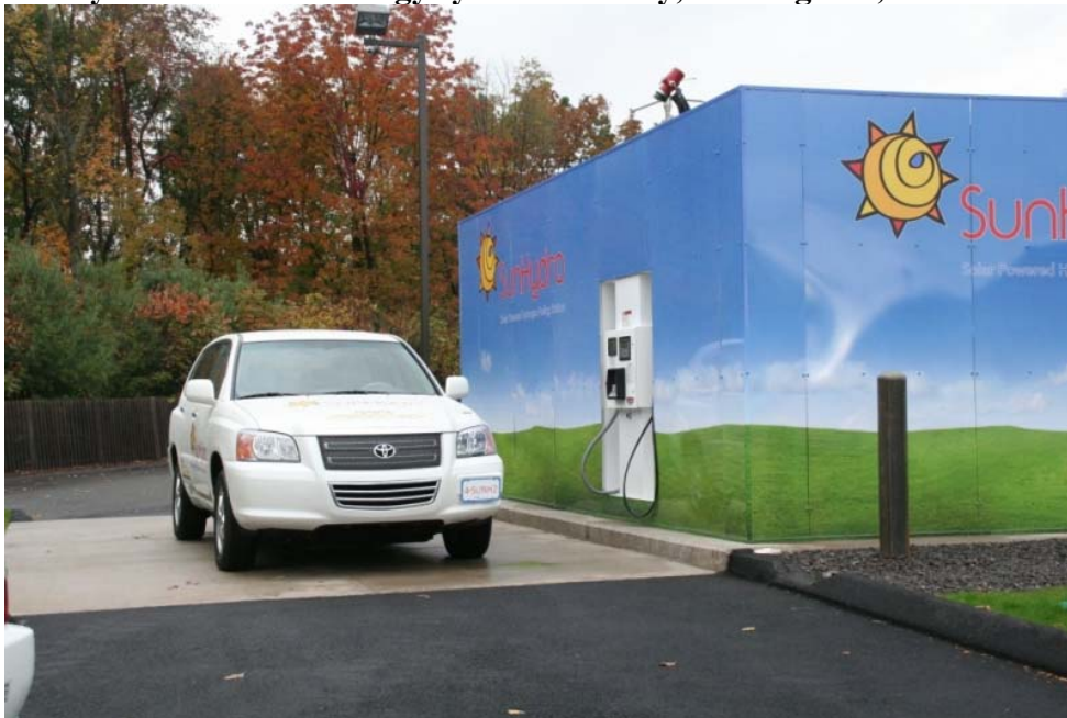
Figure IX– Hydrogen Refueling Station Infrastructure SunHydro at Proton Energy systems Facility, Wallingford, CT
