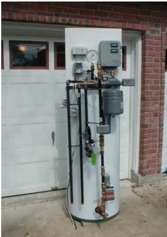
Figure A3. Water heater used for thermal recovery at Robins AFB.
