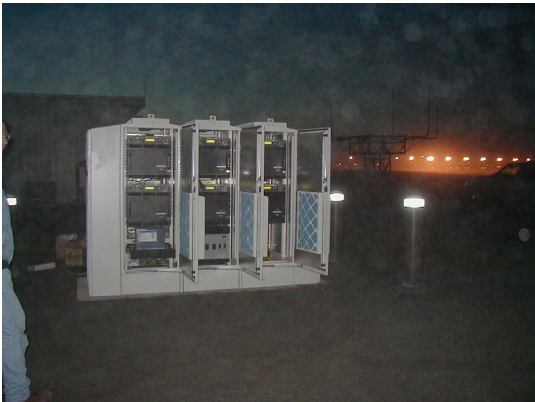
Figure A2. Fuel Cells in outdoor enclosure installed at McChord AFB.
