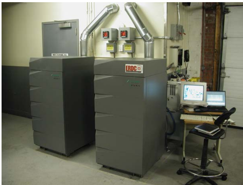
Figure A5. Two fuel cell power plants installed at the U.S. Coast Guard, Aids to Navigation Team in Bristol, RI.
