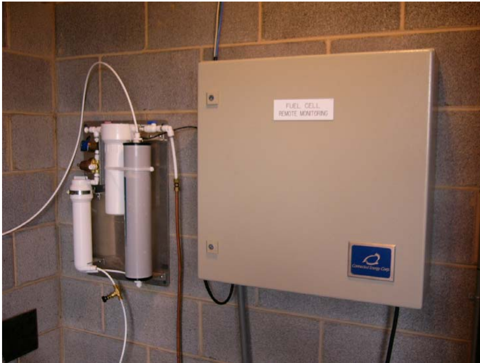
Figure A1. Water filtration system and communication and data acquisition box at Fort Gordon.
