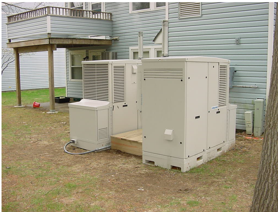
Figure A4. Two 5-kW fuel cells installed at Saratoga Springs.
