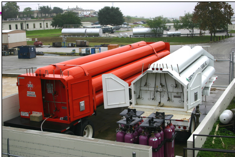
H 2 and He Tube Trailers (Revetment)
