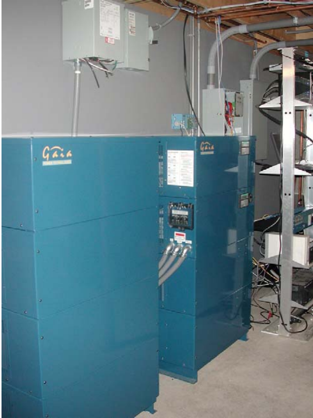
Figure 2. Residential Energy Storage Towers Fed by 5-kW Fuel Cell
